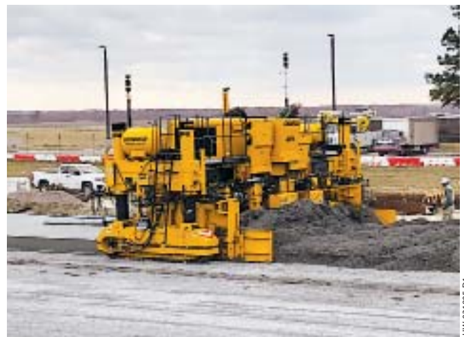
This GOMACO GP4 two-track paver with 3D machine guidance slipforms an airport taxiway at 25 feet (7.62 m) wide and 22 inches (559 mm) thick.
