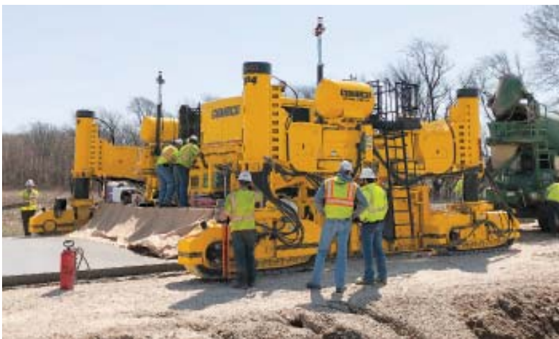
This GOMACO GP4 four-track paver with 3D machine guidance slipforms a country road 26 feet (7.92 m) wide and is equipped with a 5400 series mold and 5400 series tie bar inserter (TBI).
