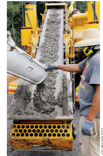
The folding conveyor features four-way hydraulic positioning for optimum concrete delivery and placement.
