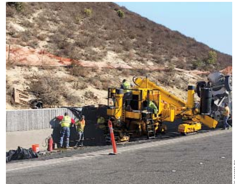
This GOMACO 3300 is slipforming a parapet wall on the left-side of the machine .
