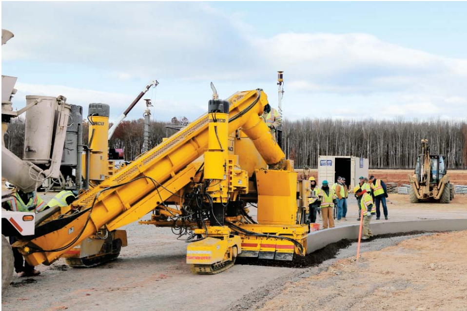
This GOMACO 3300 is equipped with a sideshifting trimmerhead and curb mold. The 3300 features the smart telescoping mold mounting system with feedback to the G+ controls for repeatable mold offset. The mold and trimmer can be hydraulically lifted over obstacles found on the job site.
